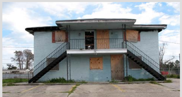
Example of a “broken windows” environment in Jefferson Parish.
