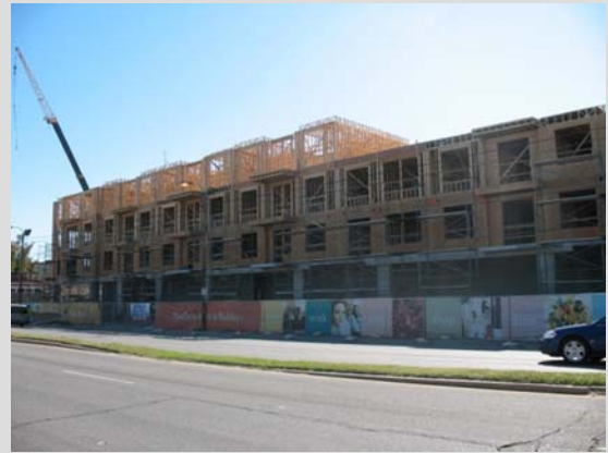
New construction must now adhere to the statewide building code.
